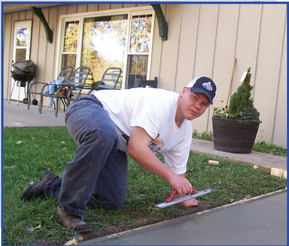
Brad finishing a concrete path at The Villages as a volunteer with his class at Kaw Area Tech.
